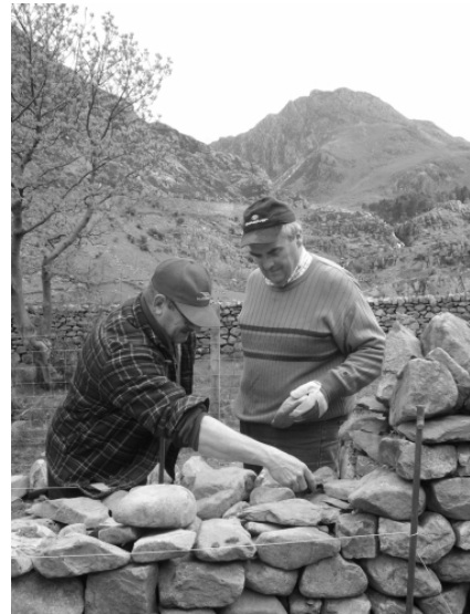
Instructor Geraint Evans (left) explains to Gwynfor Jones from Brynsiencyn how to stabilise a building stone. Blaen y Nant Taster day. © S Adcock
