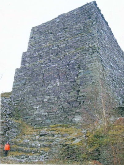
This 'Pyramid' at Dorothea stands around 12m tall on a 4m footing and is showing serious cracking
